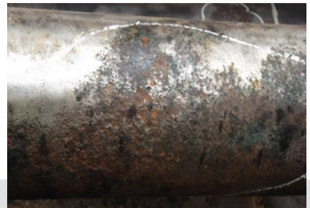
Figure 1 Typical Corrosion Found
