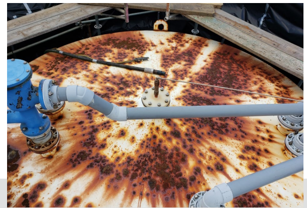
Figure 1 Tank Roof Before Composite Repair
