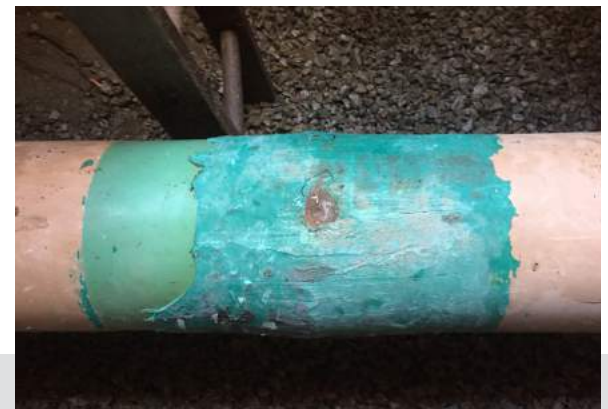
Figure 1 Damaged Girth Weld Protection System with Spot Corrosion
