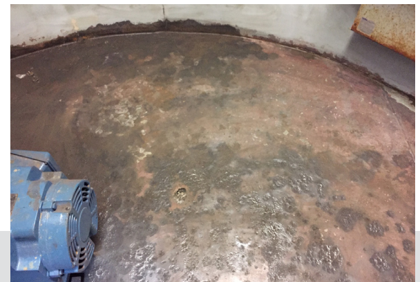
Figure 1 Extreme Corrosion with Through-Wall Failures After Surface Preparation
