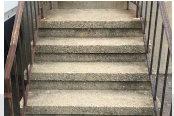
Figure 1 Staircase showing degradation and wear
