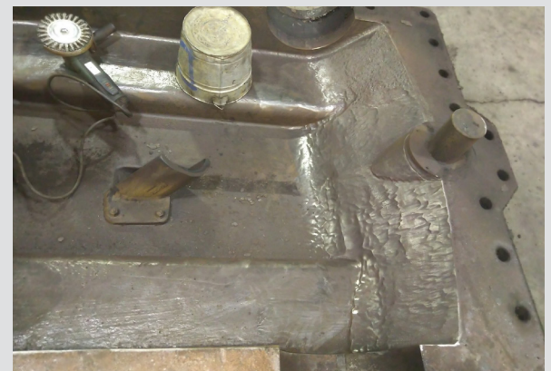
Figure 2 Close-up of Extreme Wear and Corrosion on Interior Surface of Door after Cleaning.
