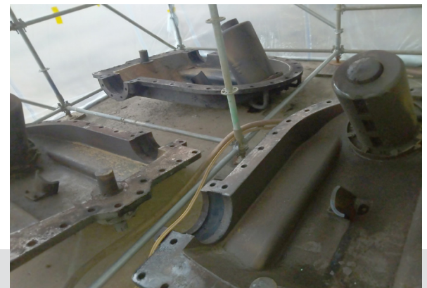
Figure 1 Pulverizer Doors Prior to Surface Preparation.
