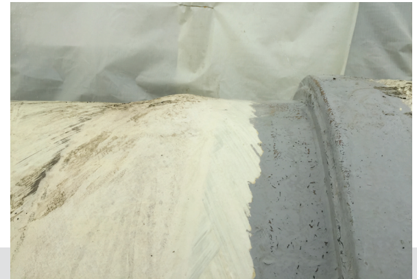
Figure 1 Close-Up of Leaking Pipe At Previous Fiberglass Repair
