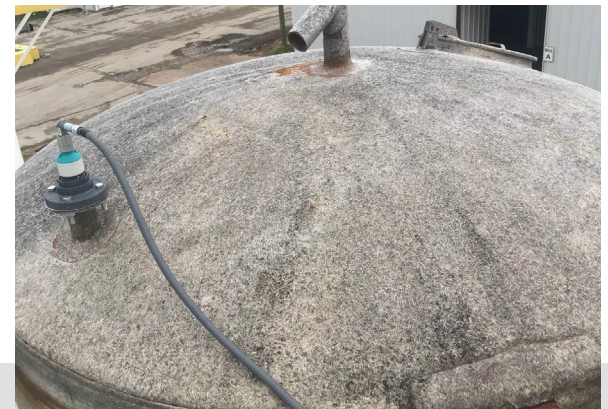
Figure 1 Close-Up View of Tank Roof Prior to Repair
