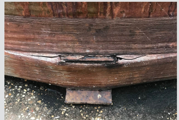
Figure 2 Cracking and Delamination of the Fiberglass at the Tank Base
