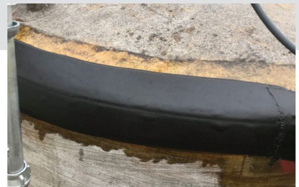
Figure 3 Carbon Fiber Repairs of the Vent Pipe, Tank Roof and Top Seam
