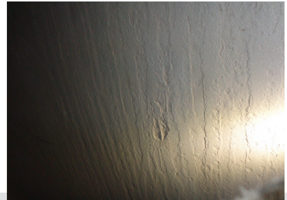
Figure 1 Severe Corrosion and Pitting on the Tank Wall After Grit Blasting
