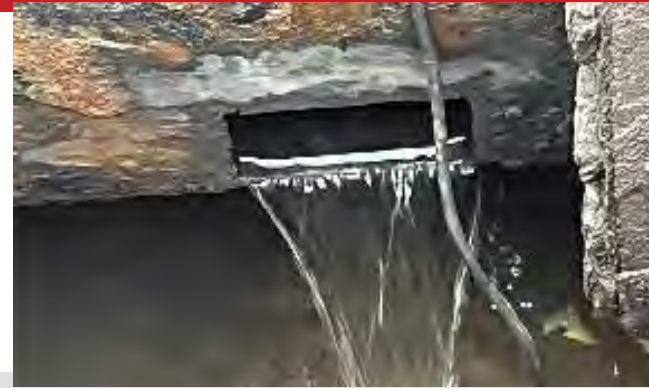
Figure 1 Identified holes in the tank were repaired with carbon fiber
