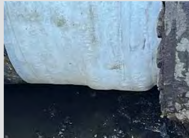
Figure 2 Repair putty filled in pitting
